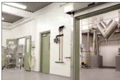
Individual and Isolated suites have separate air handling systems.
